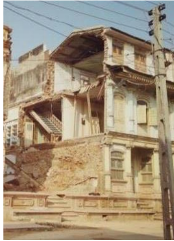
Figure 7. Dilapidation of the Bohra Haveli ( Source: Authors )
