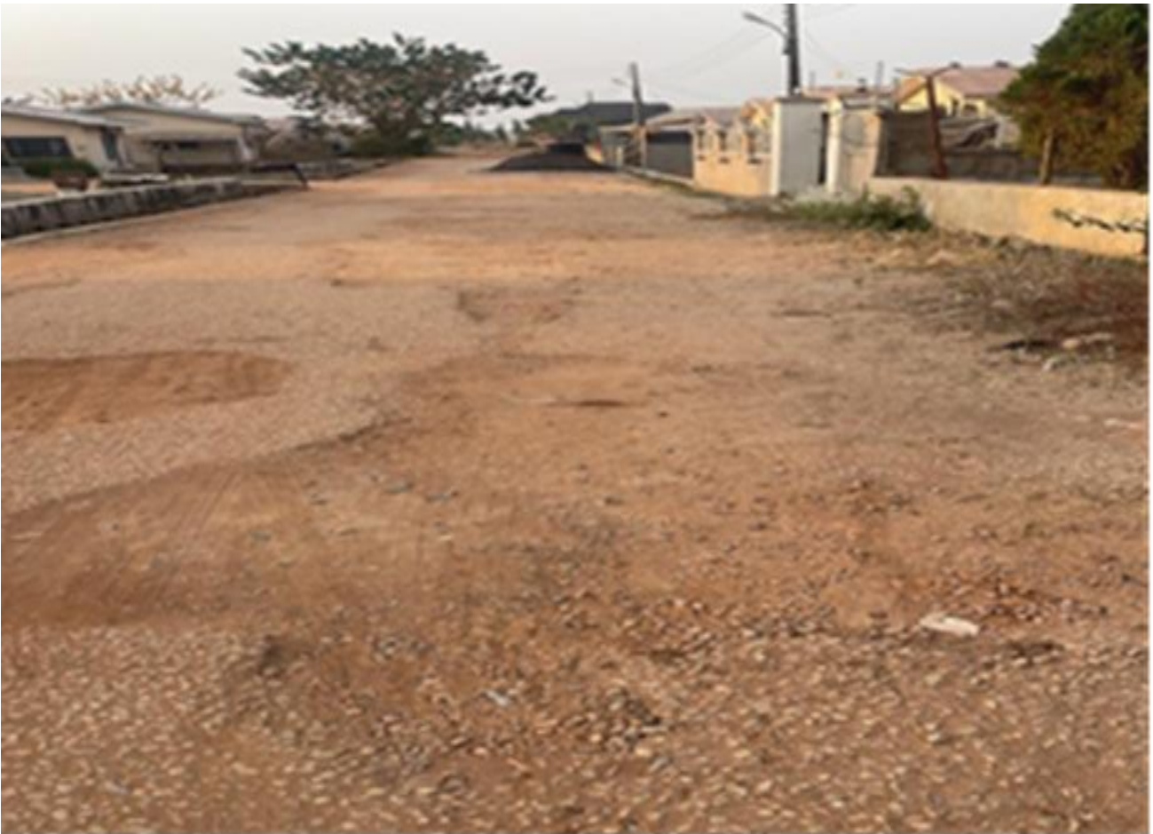
Plate 1: Road and drainage state of maintenance in Royal valley housing estate
