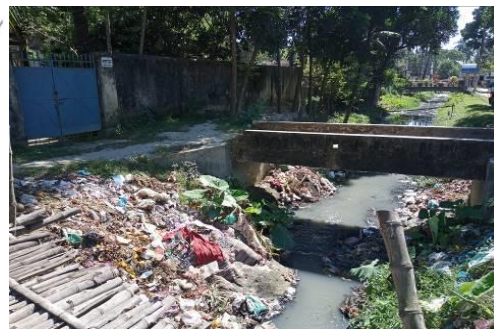
Figure 12. Garbage Disposal in Canal side.
